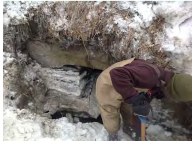
A UVM Engineering student prepares the culvert for the LIDAR scan by clearing away snow from the entrance. (Image property of VTrans)
